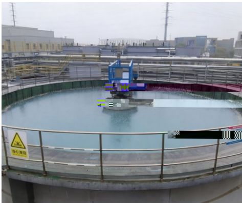
Physicochemical Sedimentation Tank
